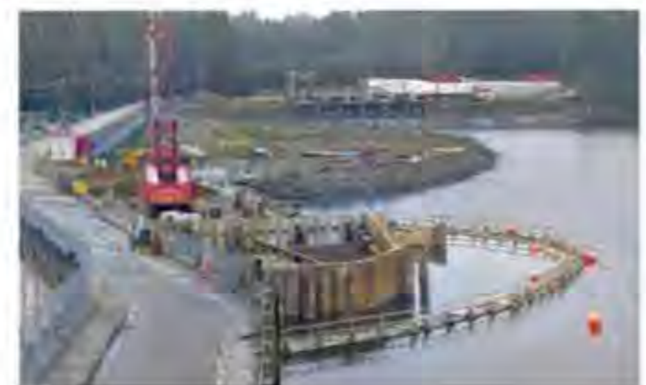
From top: Start of the Service Tunnel, in January 2015; ASL-JV's Project Manager, Scott Marshall, with BC Hydro's Stephen Watson; Close up of the cofferdam works
